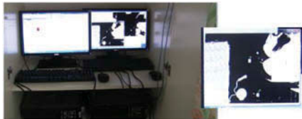
(c) Main server and vision-based tracking server in the wardrobe.
